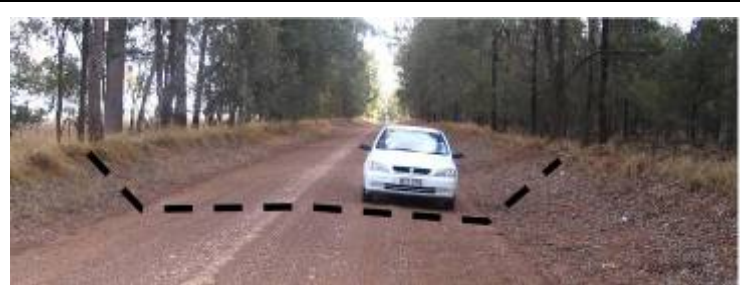
Figure 14—Incorrect road maintenance can lead to subsurface roads from which runoff can't escape.
